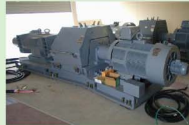
150kW rotating type generator (simulates WP, Co-generation)
